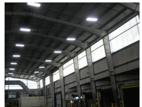
A lighting upgrade improved efficiency and quality at our plant in Berea, USA
